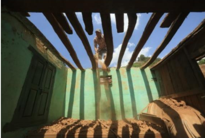
Recovery work in Kathmandu Valley following the 7.8 magnitude earthquake that struck Nepal and northern India in April 2015. A PDNA for Nepal was released in a record six weeks after the disaster; the report informed a recovery strategy and extensive global support. Photo: Laxmi Prasad Ngakhushi/UNDP Nepal/2015)
